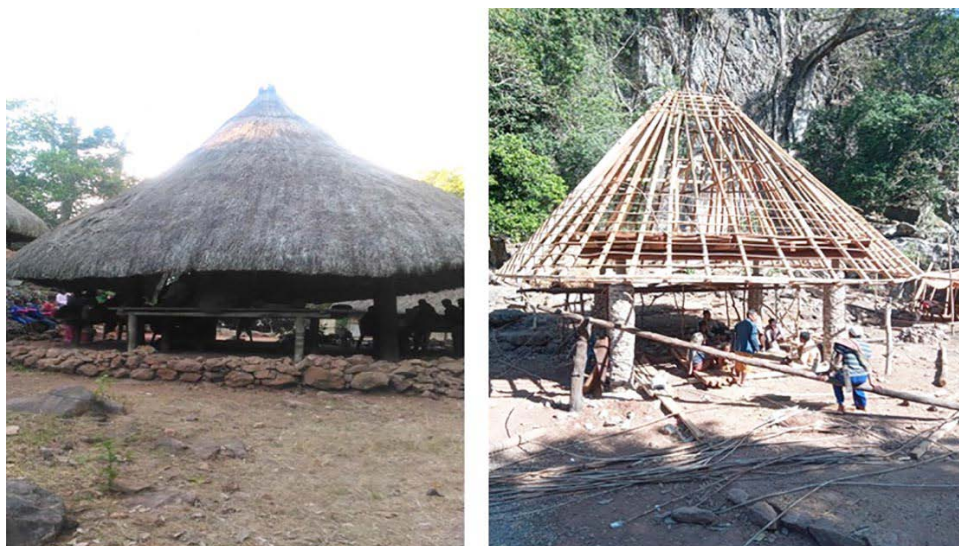
Figure 1. Lopo building and its construction in Tamkesi Village, North Central Timor Regency.
